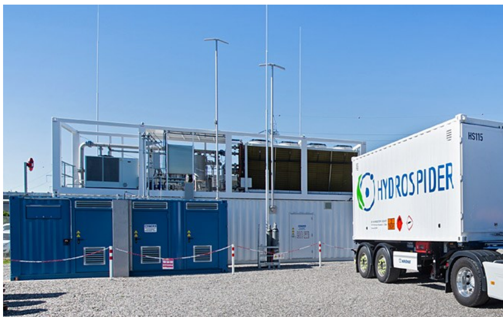
The electrolysis plant produces hydrogen from electricity generated by the Gösgen hydropower plant. Photo: Jean-Luc Grossmann
