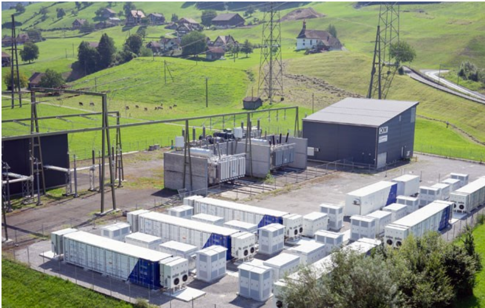
The battery storage unit in central Switzerland has a power of 20 MW.
