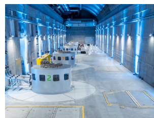
One year of successful operation: the Nant de Drance pumped-storage power plant.
